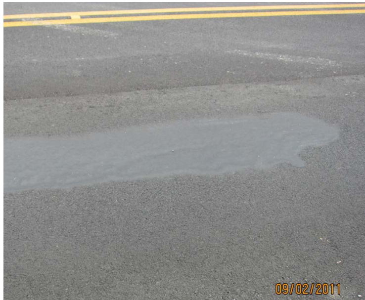
Excessive Fat Spot in new asphalt pavement.
